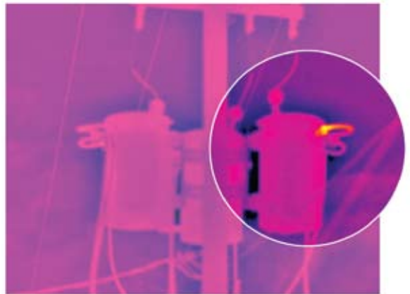
Above, a hot spot, or potential trouble spot, is detected by a special infrared camera. Each year, we use the camera to inspect more than 4,000 miles of neighborhood power lines. In addition, thousands of miles of additional power lines are inspected annually by helicopter and foot patrols.
